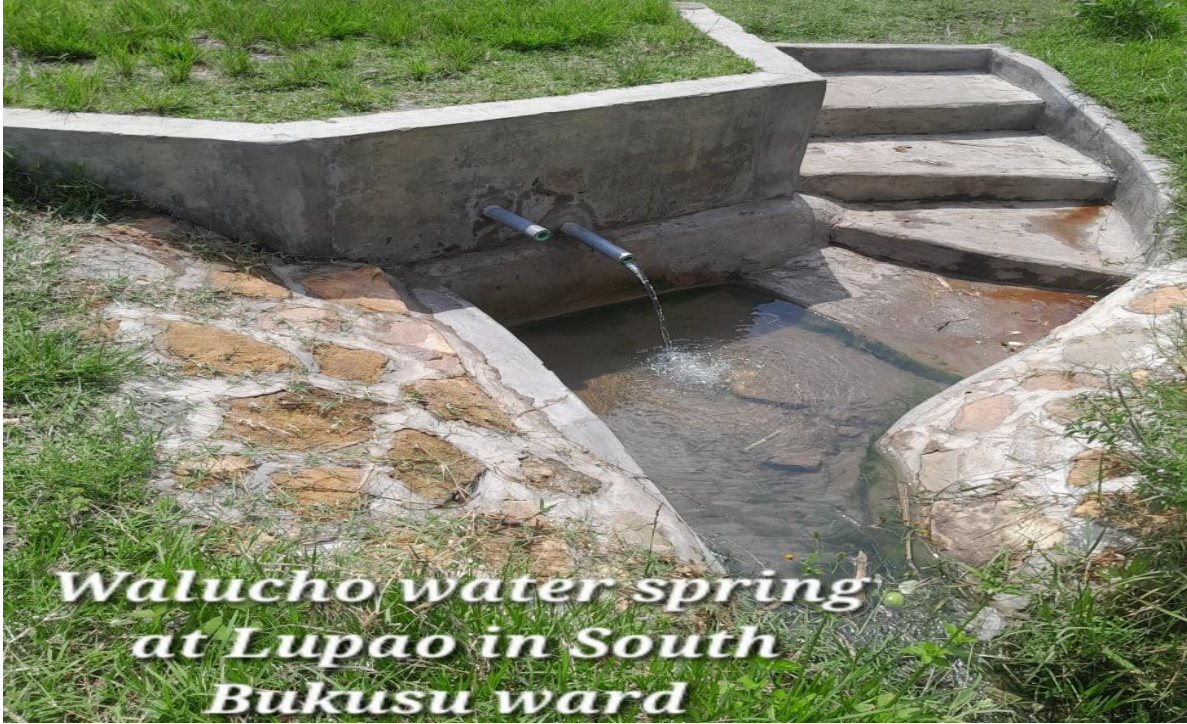
Protected Walucho water spring in South Bukusu ward
