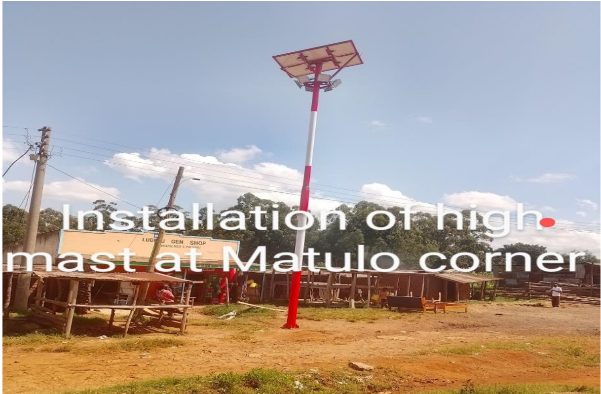
High mast floodlight at Matulo corner, in Matulo ward
