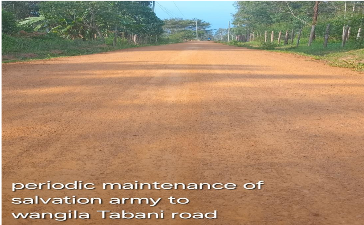
Routine maintenance of Salvation Army to Wangila Tabani road in Ndalul Tabani road
